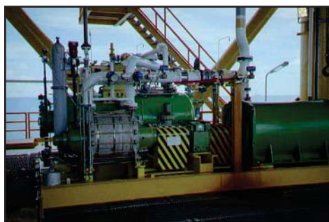
NASH 2BG Compressor used for vent gas compression on an offshore rig
