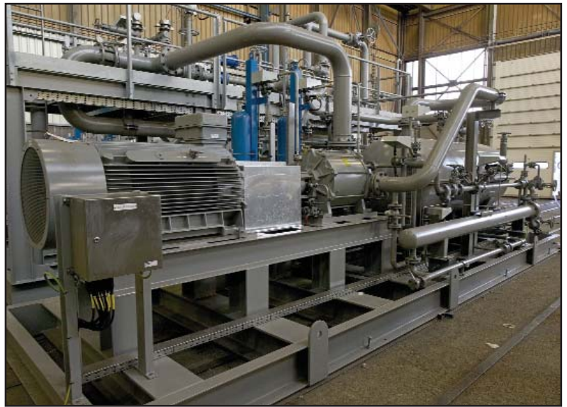
XL350 Vent Gas compressor system
