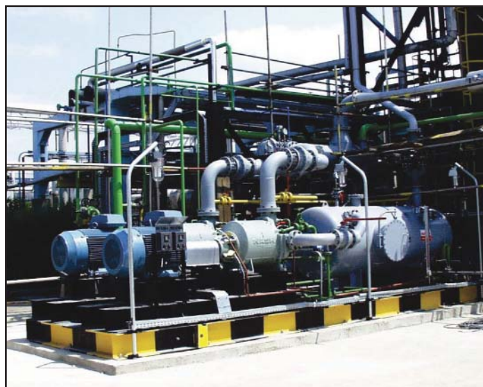
Duplex vacuum system used on a crude oil distillation tower
